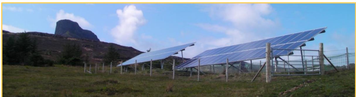
Figure 1. Off-grid energy system on the isle of Eigg, June 2008
